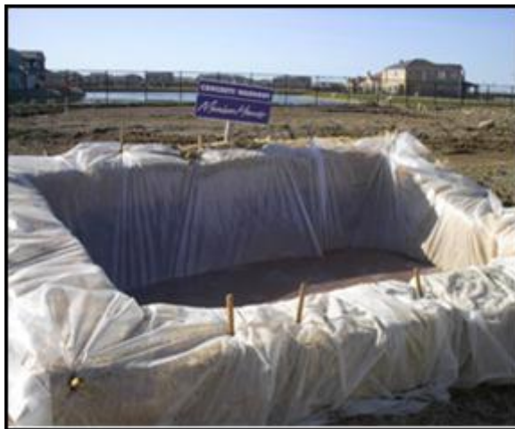
Figure 4 Example of a Turkey Nest Concrete Washout Pond (County of Lake, California, N.D.)
