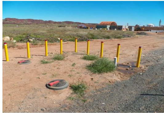
Picture of Sanitary wastewater spill
