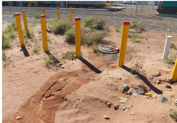
Picture of Sanitary wastewater spill
